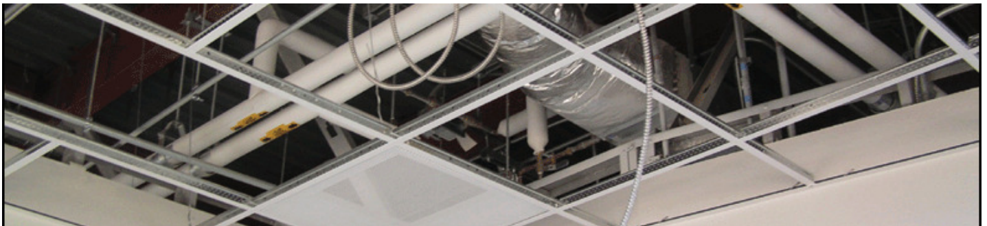
The ceiling grid is the single most important structural aspect of a modular cleanroom – make sure it remains true and level and that all components are functional, as well as properly seated and sealed. Photo courtesy of Technical Air Products.
